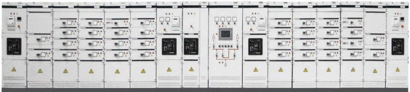
“Freecon ST” Low Voltage Electrical Switchboard, (7,000 A max.), “SIVACON S8” form factor, manufactured by “NIPOM” OJSC under Siemens’ license
