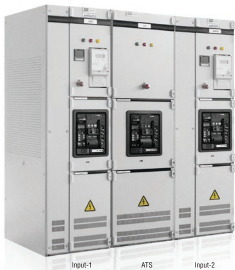
"Freecon" Low voltage Electrical Switchboard (lead-in section)
