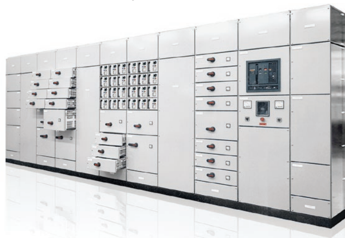
“Freecon SM” Low Voltage Electrical Switchboard, (8,500 A max.) Logstrup form factor, manufactured by “NIPOM” OJSC under Logstrup’s license
